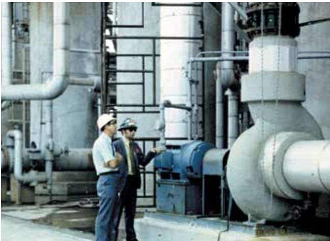
A 3175 installed in a major chemical plant.
